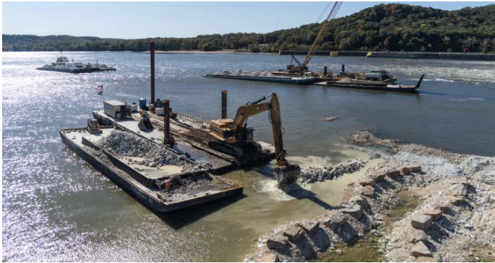
Since May, contractors have been meticulously placing rocks in a wave-like pattern beneath the spillway at Lock and Dam 22. This innovative design is part of the first-ever fish passage on the Upper Mississippi River, a project aimed at enhancing aquatic connectivity and ecosystem health. Photo by Joe Stadele, J.F. Brennan Company, Inc.
