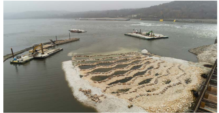
For the first and final time, the wavy rock weirs below the spillway at Lock and Dam 22 are fully visible. Once the coffer dam is removed and the Fish Passage Project becomes operational, these structures will be submerged, quietly supporting the river's ecological balance. Photo by Joe Stadele, J.F. Brennan Company, Inc.
