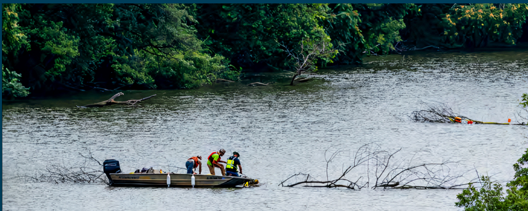
A boat crew for the Pittsburgh District attaches tree bundles to concrete blocks submerged in a water basin near the Montgomery Dam on the Ohio River in Monaca, Pennsylvania, Aug. 8. (Photo by Michael Sauret)
