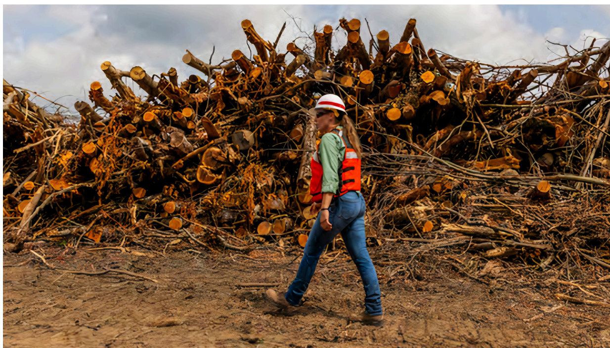
Jenna Cunningham, resident engineer for the Montgomery Locks and Dam construction with the Pittsburgh District, walks through a site being cleared for a concrete batch plant in Monaca, Pennsylvania, July 20. Some of the trees cut down were repurposed into fish habitats. (Photo by Michael Sauret)
