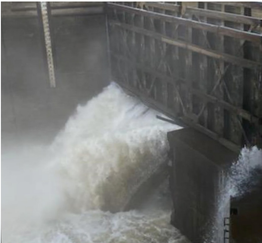
Water pours into Demopolis Lock after concrete failure in a miter gate sill.
