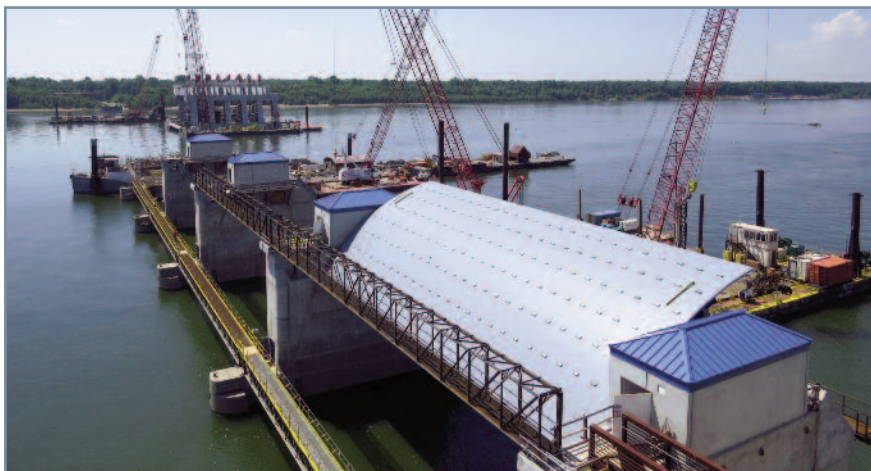
Olmsted's tainter gate #1 is shown (on right, raised), with the catamaran barge setting Paving Block 5 (in distance, back left), performed on June 10, 2015.
