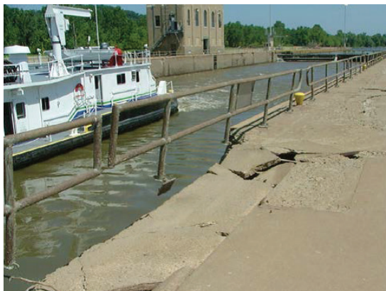
Collapsing lock wall at LaGrange Lock on the Illinois Waterway.
