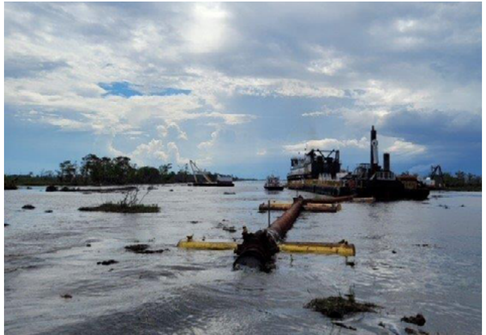
Hurricane Ida, with its more than 150 mph winds that resulted in scattered debris as shown, made it the second most damaging storm to the state of Louisiana behind Hurricane Katrina. Here, a drag line crane removes vegetative and other debris ahead of the cutterhead dredge.
