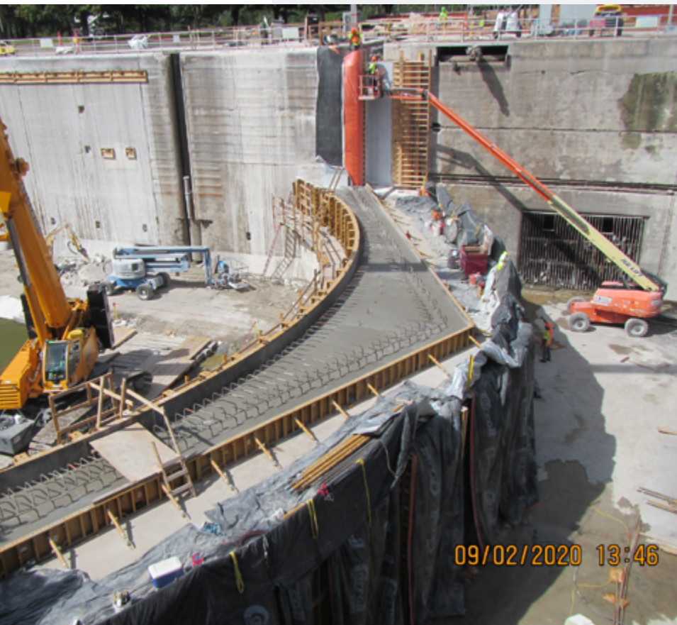
The first concrete is placed on top of the upper gate sill at Marseilles Lock.
