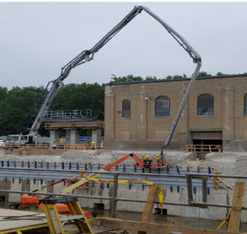
Precast panels are installed at LaGrange. Photo credit: U.S. Army Corps of Engineers.
