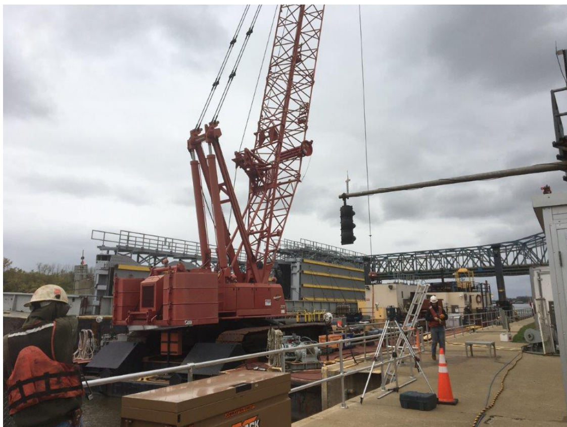
Eight lock and dams sites on the Illinois Waterway need repair.
