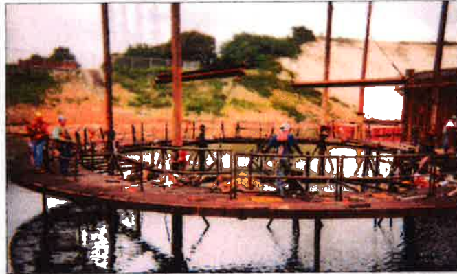
Above: The template construction workers used in 1993 to begin constructing the cells of the cofferdam.
