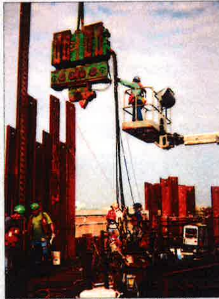
Above: A pile driver or vibro hammer is lowered by crane and placed on top of the steel in order to drive it into the riverbed, a job Richard Berry, of Metropolis knows all about as he was a pile driver foreman when he first began in 1993. He worked on the Olmsted project for a total of eight years.
