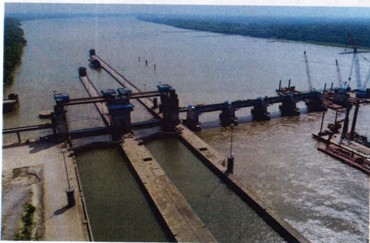
The Olmsted Locks and Dam project, originally scheduled for completion in 2008, will officially open to commercial vessel traffic in October. This aerial photo from July 2017 shows construction continuing on the Ohio River dam and its wickets, with the lock chambers at left.
