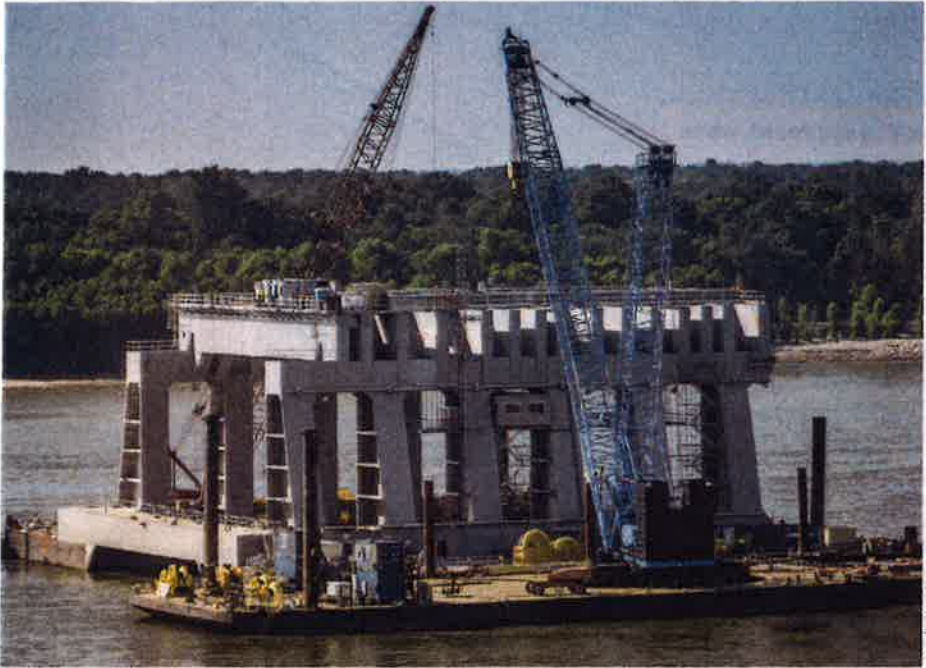
Crews at Olmsted in late July dismantle the world's largest catamaran barge, which was purpose-built for the "in-the-wet" method used to construct the new dam. Massive concrete sills were precast on land, then transported on the river to be set into place.
