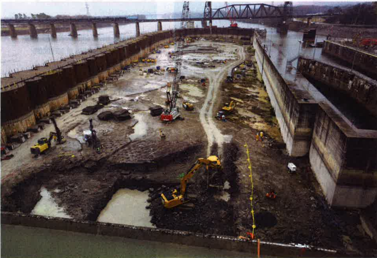
Work continues in the cofferdam at the Chickamauga Lock Replacement Project in December 2017. The Water Resources Development Act of 2018 includes a change report for the Tennessee River project that ensures continued construction after original funding has been spent. The earliest estimated completion date for the $760 million lock is 2024.
