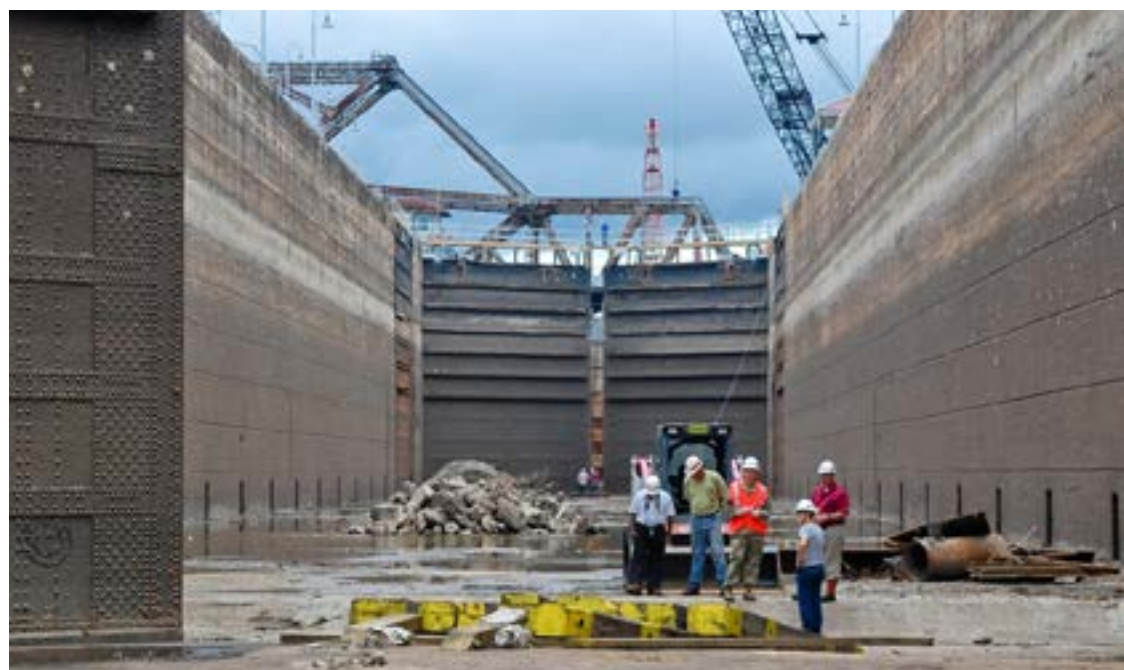
Corps personnel stand in an empty lock chamber during the maintenance and dewatering project of the Inner Harbor Navigation Canal completed by the U.S. Army Corps of Engineers during 2016.
